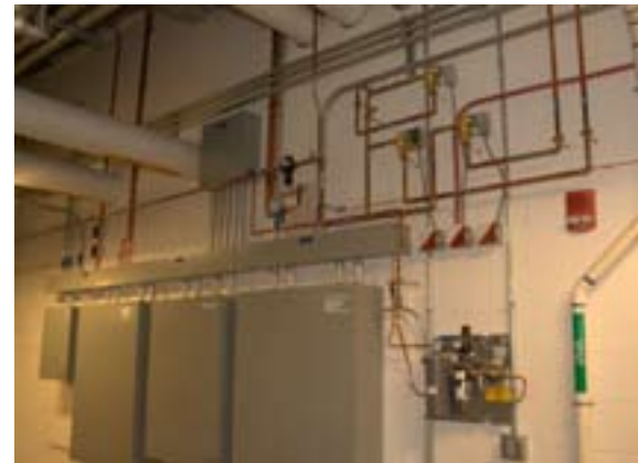
The control cabinets and pneumatic air systems are utilized as part of the buildings DDC control system. This system allows the University to see and adjust the building HVAC systems from a remote location.
