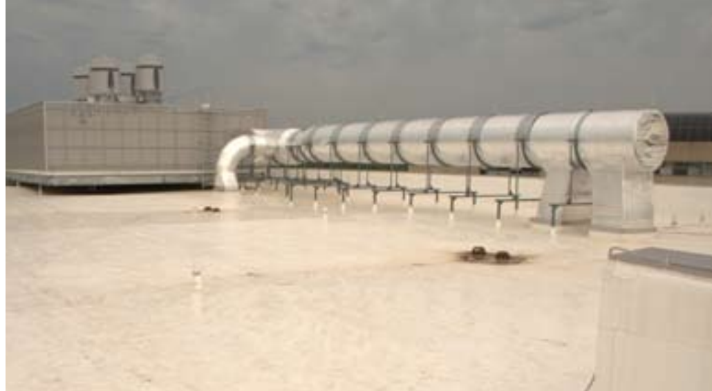
The roof mounted duct system, penthouse and exhaust fans. Warm building air is exhausted through a heat recovery system which then preheats makeup air for the building. This type of system is normal on LEED projects, as it reduces building operating costs.
