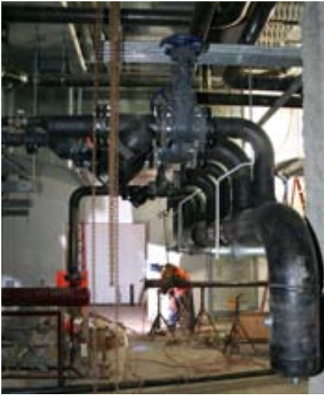
The steam header serves the building's hydronic and domestic hot water systems. ACI prefabricated most of the welded pipe systems offsite.
